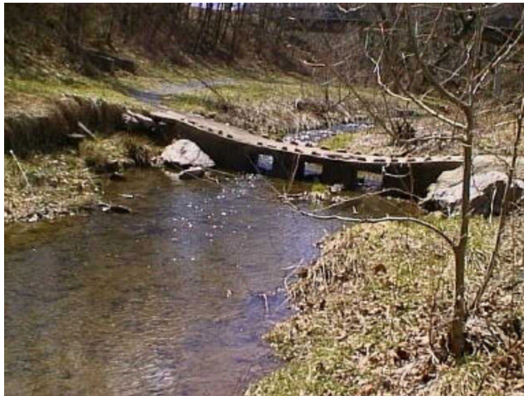
Figure F-7. Inadequately designed/ constructed stream crossing
