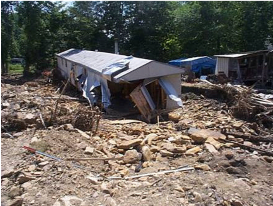
Figure 1-4. Example of Flood Damages in July 2001
