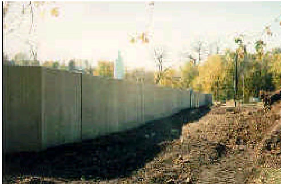
Figure L-5. Floodwall protection structure
