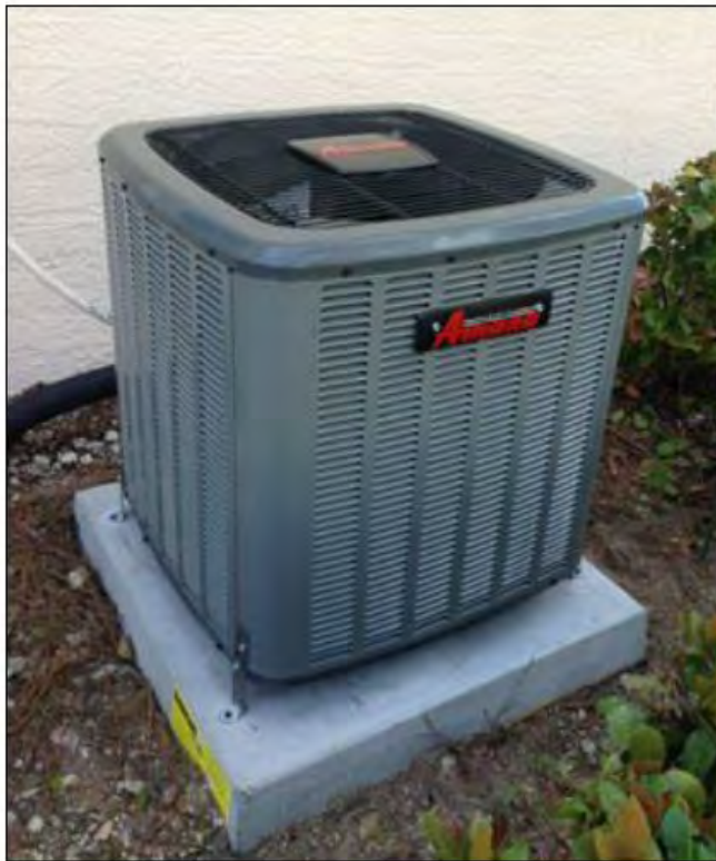
Heating and/or Cooling
