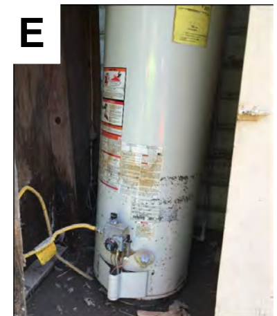
Electric Water Heater
