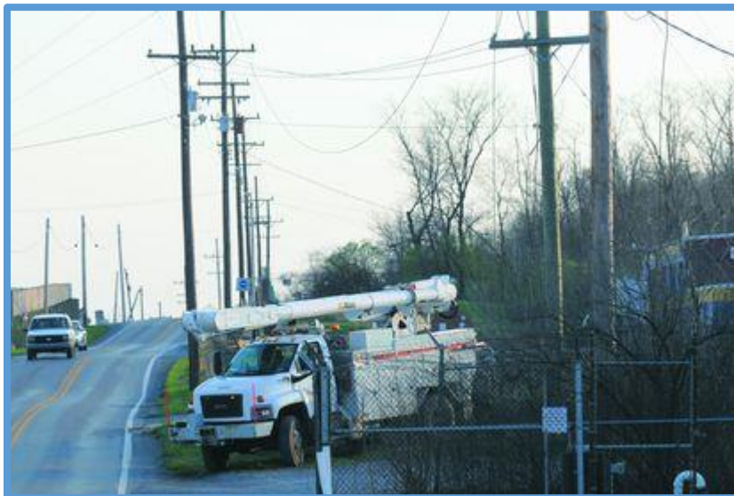
Figure 4.3.20-1 Crew Repairs Damage from Transformer Fire in Berkeley County 3/26/16 (Agnir, 2016)
