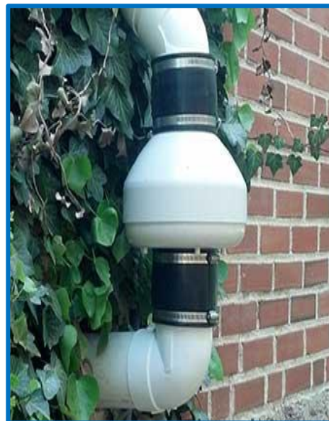
Figure 4.3.10-5: Radon Mitigation Fan Installed on Commercial Building in Martinsburg (SWAT Environmental, 2015)
