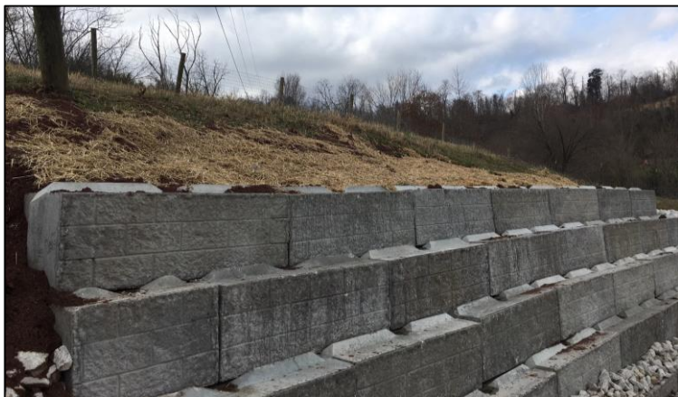
Retaining walls that allow proper drainage can reinforce slopes (photo by WV Dept. of Transportation)
