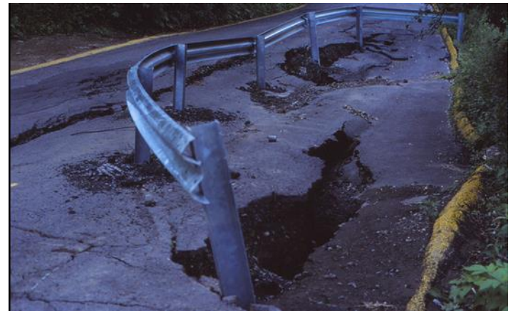
Cracks in paved surface (photo by J.S. Kite)
