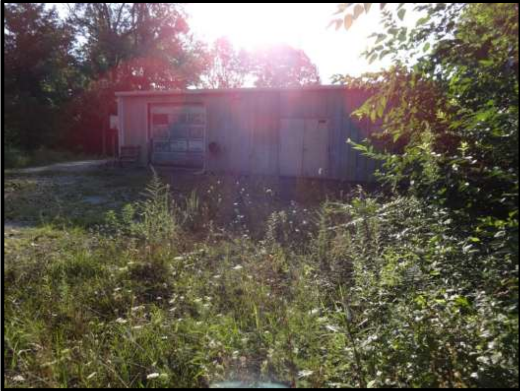
Photo 4: Back view of commercial building facing southeast. Picture taken from near open channel. Building located along overbank of tributary to Mill Creek
