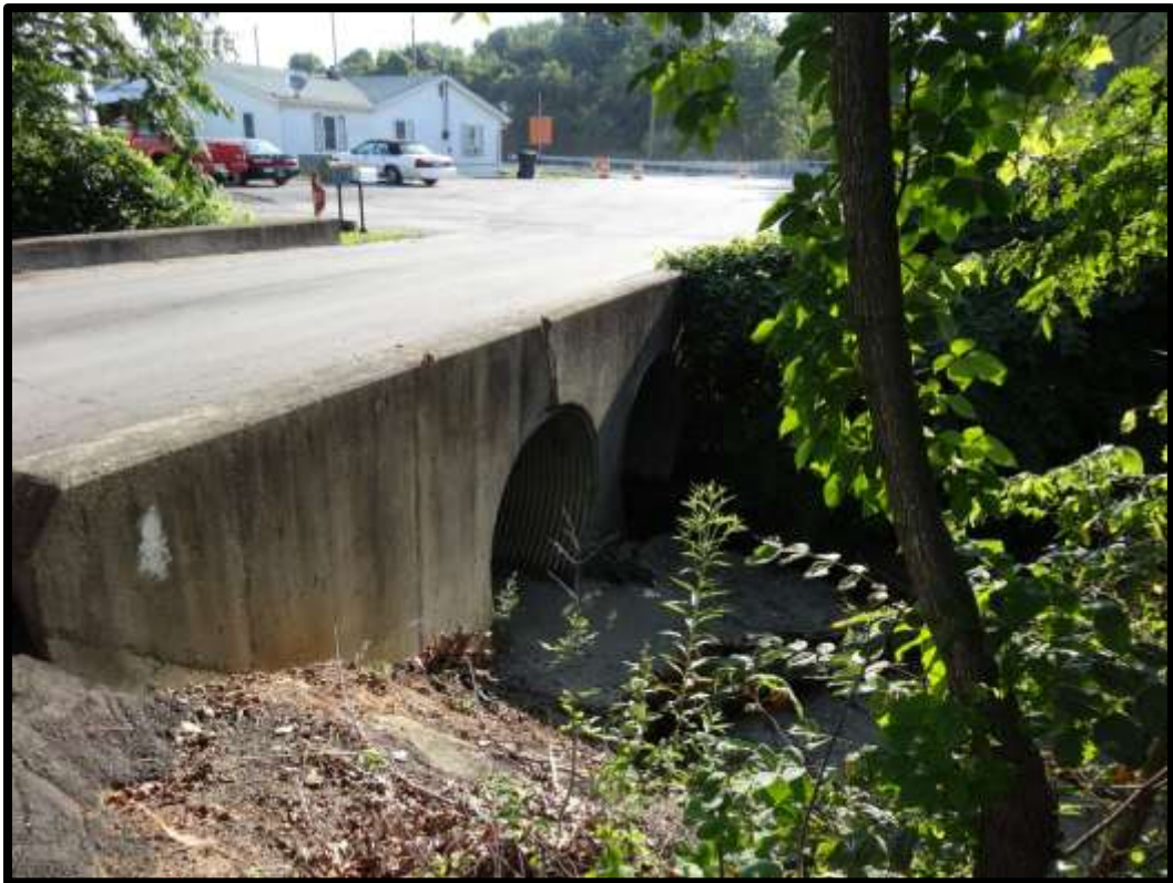
Photo 5: Drive entrance culvert at southern edge of study area; potential for debris accumulation.
