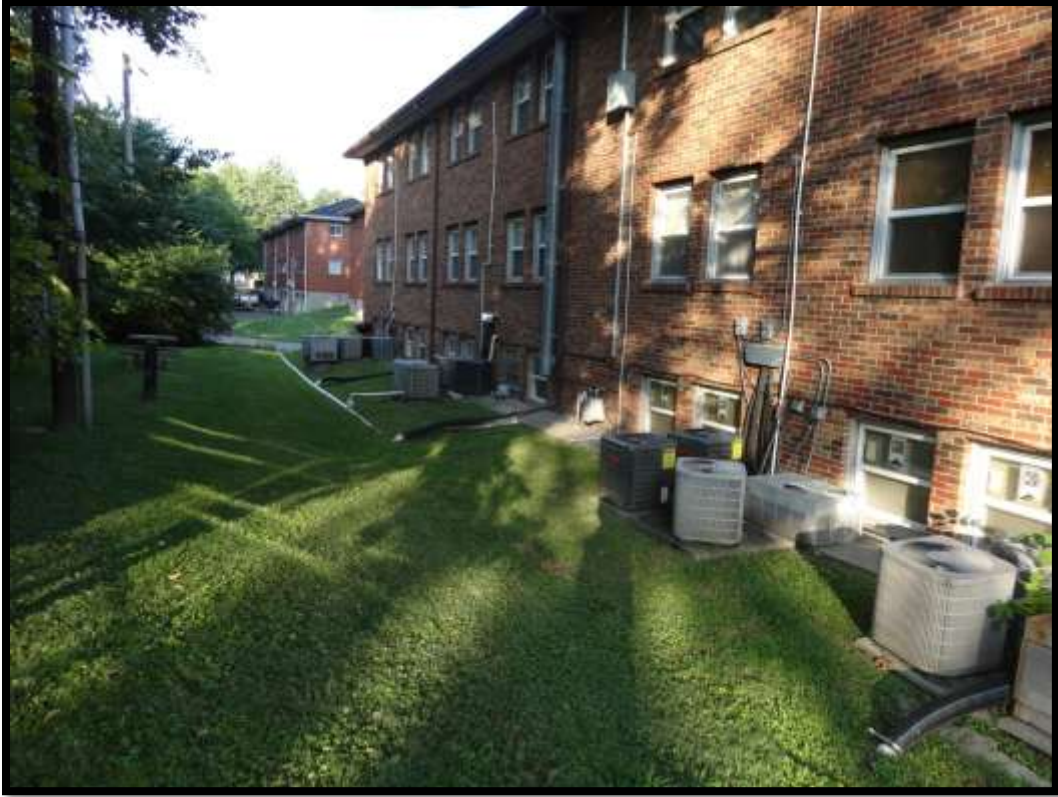
Photo 4: Perimeter drainage of middle property, designed to convey water away from building.
