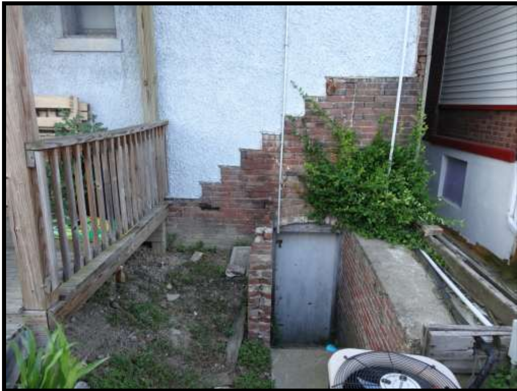
Photo 2 – View of back of building in RL area, facing SE. Doorwell is below ground elevation.
