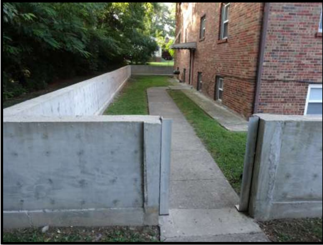
Photo 2: Floodwall installed at the back of the easternmost property.
