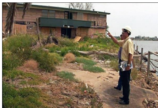
Figure 7-3: Screening the exterior of a damaged structure
