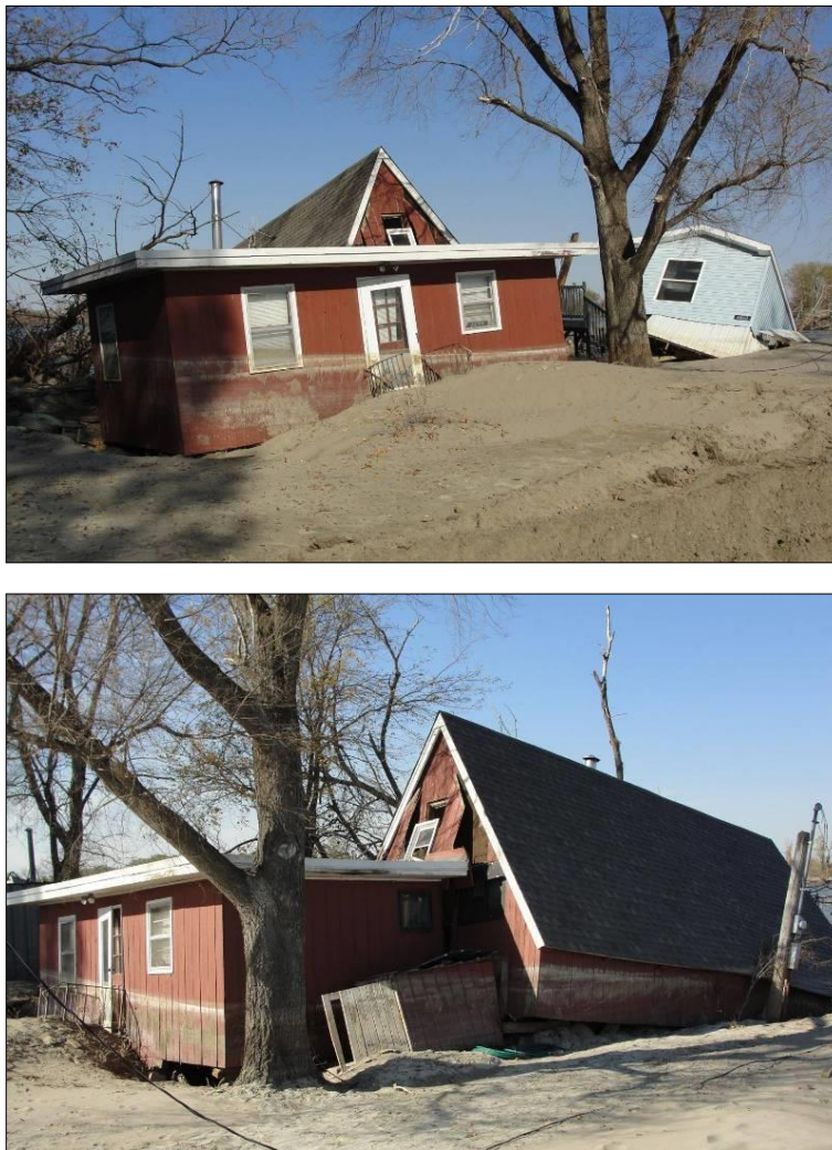
Figure 9-1: Two views of the same structure showing a high water mark, structure displacement, and some of the damage
