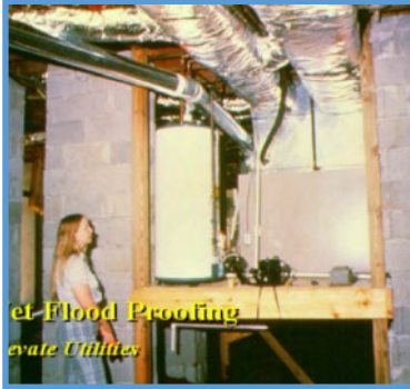
Elevated HVAC / WH (Interior)
