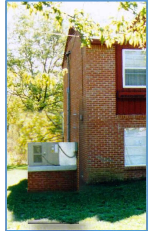
Elevated HVAC (Exterior)
