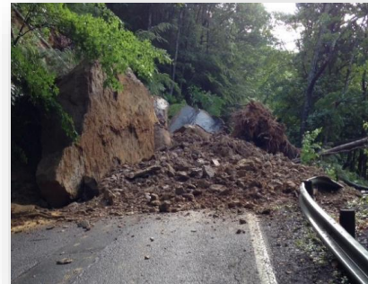
Landslide Risk #2 WV Hazard
