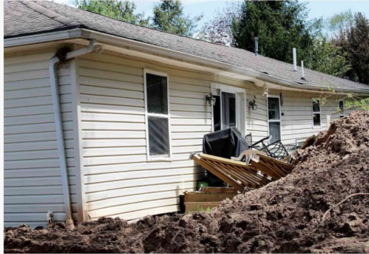
A landslide Sunday evening damaged a Washington Bottom home and forced the evacuation of several neighboring houses. (Photo by Michael Erb)
