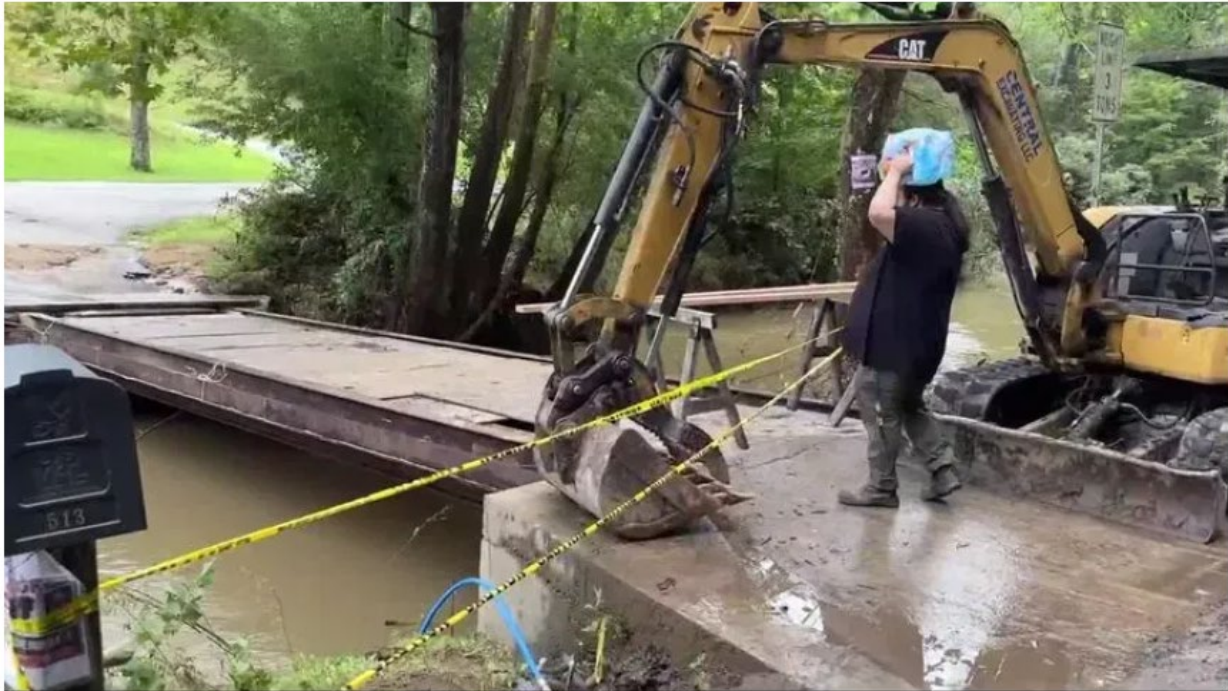
A bridge to the Fayette County Animal Shelter is damaged by severe weather. (WCHS)
