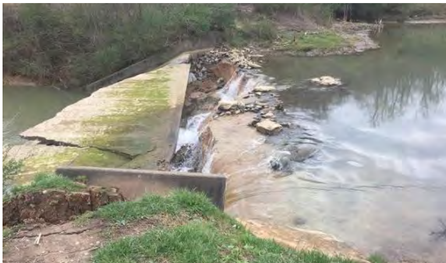
Auxiliary Spillway Failure
