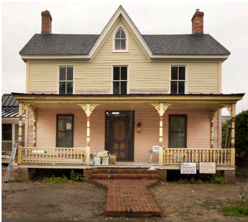
This home was elevated as part of a rehabilitation project. Concrete block piers were clad in brick for a more historically appropriate appearance.
