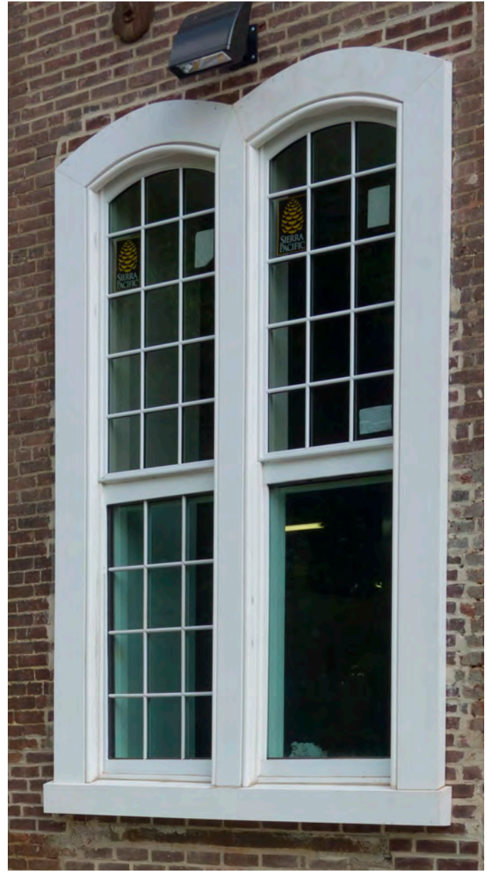
As viewed from the exterior, the replacement sash with the aquarium glass looks similar to a typical replacement window with applied muntins, with a slight difference occurring at the meeting rail, where the offset between the upper and lower sashes is minimized.
