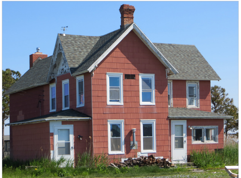
Figure 2.27 - Historic building in floodplain that would benefit from minor maintenance. Dorchester County.
