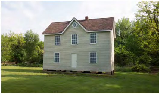
The Henry Wilson House was elevated on brick piers. The front stair has yet to be installed.
