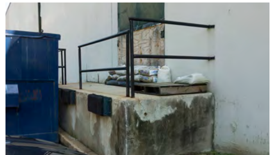
"Temporary" flood protection can be found on this rear door at the Meadow Mill.
