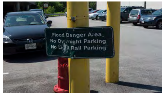
The parking area is repaved approximately every 3 years at the Meadow Mill due to flood-triggered subsidence.
