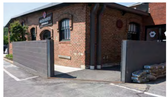
Following loss from a 2014 flood, the window sills were raised and flood walls installed at the Meadow Mill.
