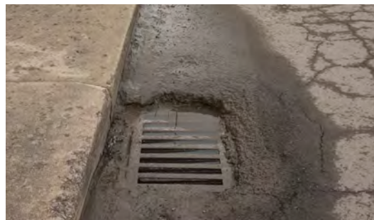
Standing water was noted at this storm drain, indicating a clogged drain.
