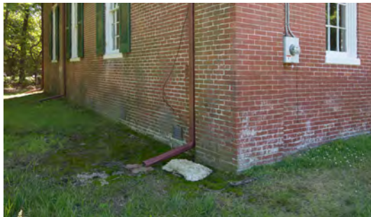
The efflorescence suggests water saturation at this Taylors Island church.
