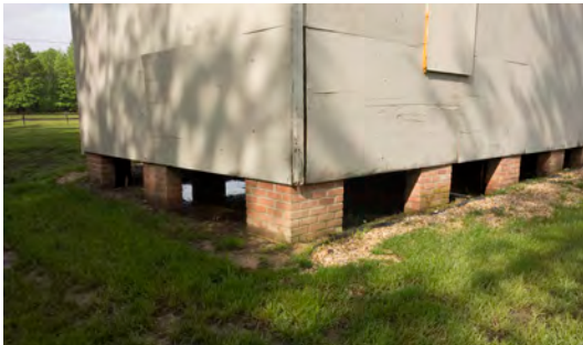
Standing water is visible under the Henry Wilson House.
