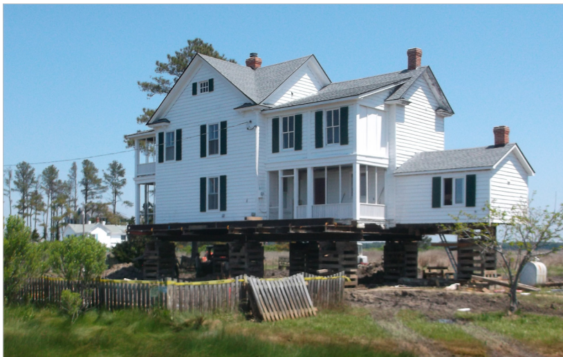
Figure 2.38- Elevation in progress of a late-19th century historic home on St. George Island, St. Mary's County. The building was elevated to the BFE plus three feet of freeboard. (Source: MEMA)
