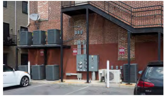
Mechanical and electrical equipment installed at grade is at risk for being damaged by flood waters.
