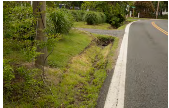
The ditches at the side of the road are not continuous.
