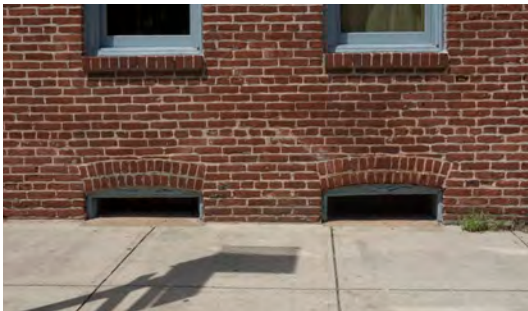
Windows can provide a path for flood water entering a basement.
