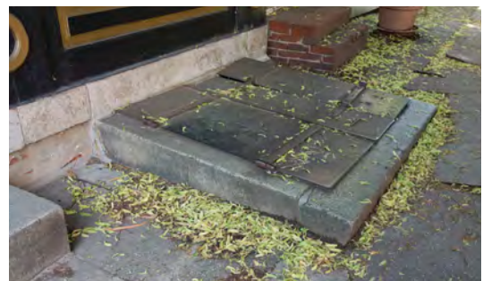
Areaways, including those that service commercial buildings, provide a path for flood water to enter a basement.
