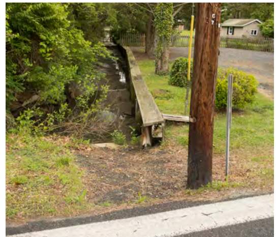
Both piped and surface storm water is directed towards this drainage channel, which often backs-up, flooding the roadway surface.
