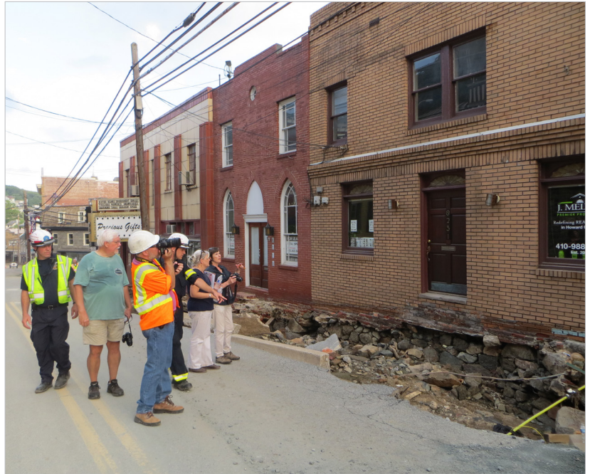
Figure 2.22 - The MHT and Howard County employees conduct damage assessments after the 2016 flash flood. Ellicott City, Howard County.
