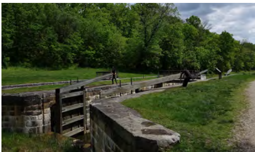
Completed work includes the restoration of Lock 44 in front of the lock tender's house.
