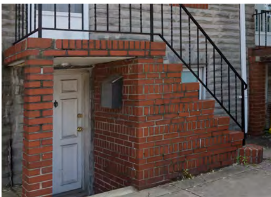
Although the primary floor is raised, the lower level, which appears occupied, is susceptible to flooding.
