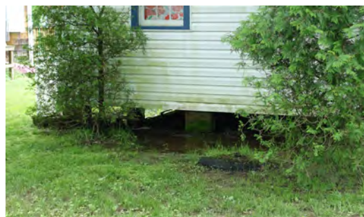
Standing water was observed at several locations, including under this building.
