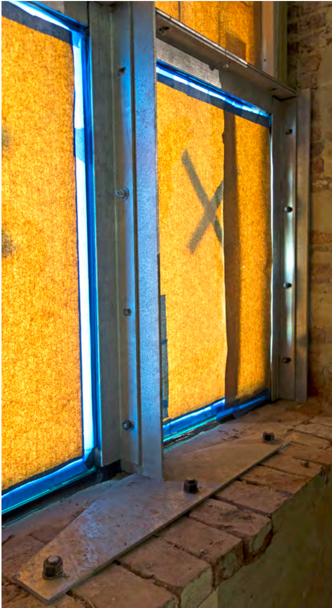
The lower sashes of the ground floor windows at Whitehall Mill are constructed using aquarium glass supported by a heavy-duty steel frame that is secured into the masonry, with a standard upper sash.
