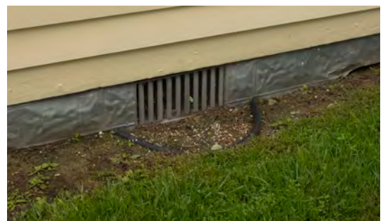
Proper ventilation of crawl spaces is important to minimize deterioration of wood floor framing.
