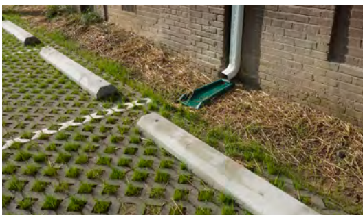
Storm water from the roof drains to grade. Also note the permeable parking pavers.
