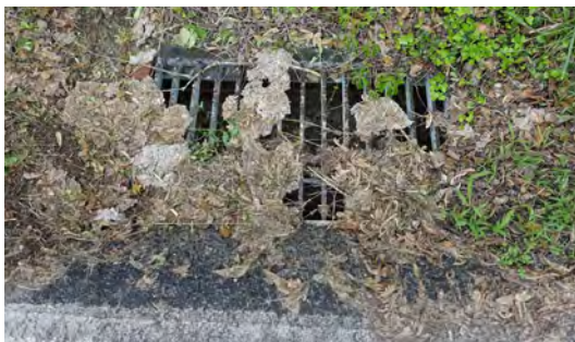
Debris was clogging some of the storm water drains, impeding water flow.
