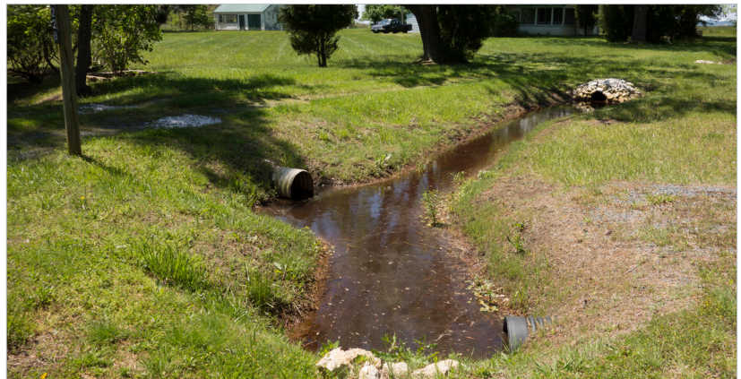
Figure 3.8 - Engineered drainage system to convey stormwater to a retention area away from historic cottages. Shady Side, Anne Arundel County.
