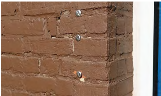
Attachments for flood gates are located at door jambs and embedded in paving.
