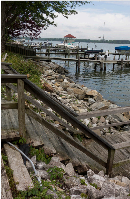
Figure 3.2 - Rip-rap shoreline protection (rocks in center of photograph) preventing further erosion of the shoreline along the West River, protecting the fisherman's village of Shadyside, Anne Arundel County.
