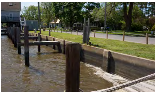
A concrete bulkhead has been installed along the river, and new houses along the water are being constructed at a higher elevation.
