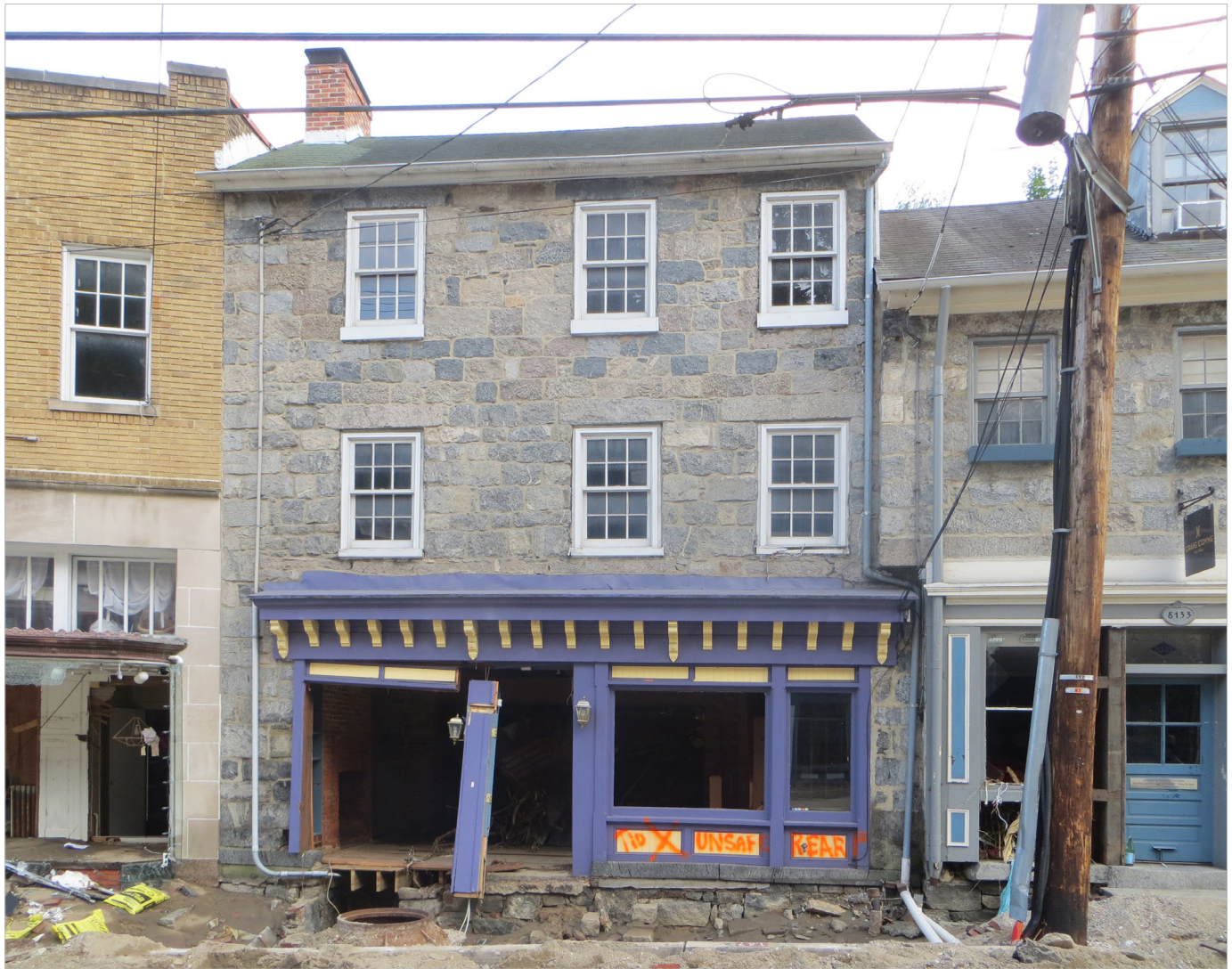
Figure 2.21 - Building Tagged as "Unsafe Rear" by an assessment team. The rear wall of the first floor was blown out due to floodwater entering the front of the building. Ellicott City, Howard County, 2016.
