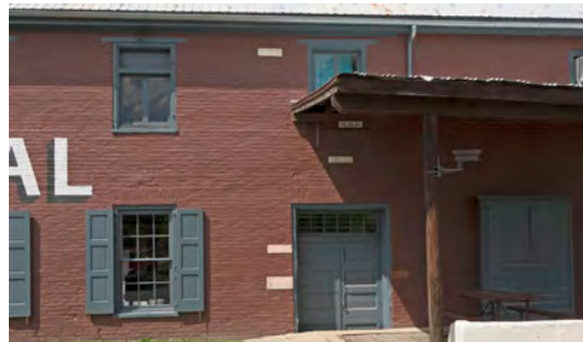
The white markers on the Cushwa building indicate the heights and dates of past flood events.
