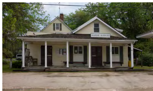
Standing water could be found in front of this store, whose first floor is slightly raised above grade.
