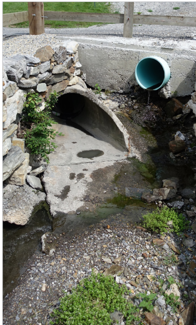
Figure 3.12 - An old outfall (left) and a potentially unpermitted discharge from a nearby property (center) that discharges into a ditch which could be retrofitted to allow for a stormwater filtration best management practice such as bioretention a swale, or a manufactured filtration device to improve water quality downstream. Williamsport, Washington County.
