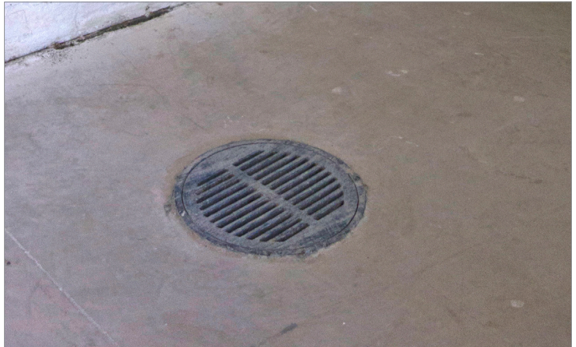
Figure 3.22 - Accumulated flood water is evacuated through floor grates and a sump pump at Mount Vernon Mill #1, Baltimore City.
