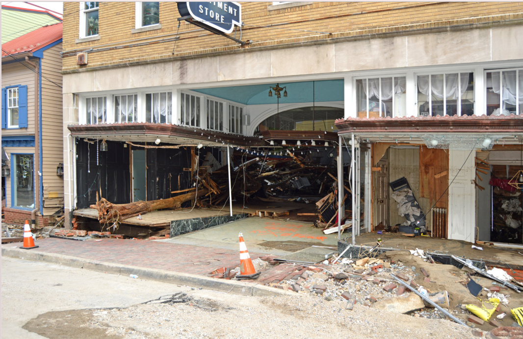
Figure 2.23 - A tree was found lodged in the storefront during initial damage assessments after the 2016 flash flood in Ellicott City. Although the storefront glazing system was lost, its cornice and the transom windows above can be stabilized and retained in the rebuilding process.
