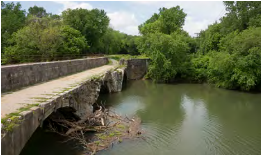
Plans to restore the aqueduct require the rebuilding of the east wall. Also note the debris in the river.
